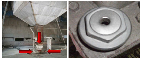
Fig. 4. The location of ash-blowing nozzles in ash delivery system (left) and view of ash-blowing nozzle (right).
